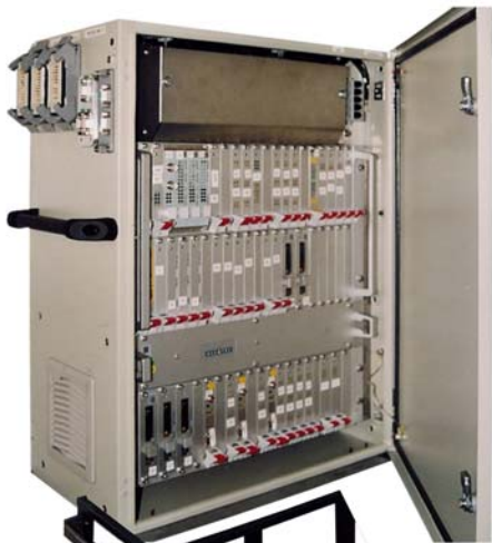
Application: Signalling control systems
