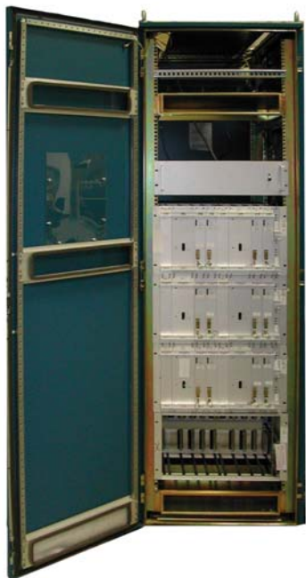
Application: Control system
